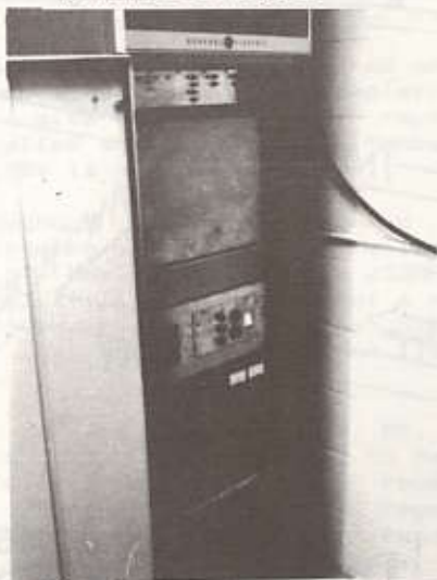
GE Mastr II cabinet interior, top to bottom: 2 meter duplexer, control panel, 2 meter repeater, 2 meter power supply, 220 repeater, 220 duplexer.
